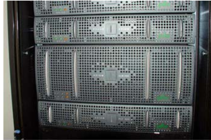
Pillar Data Systems Axiom 500 7TB SAN
